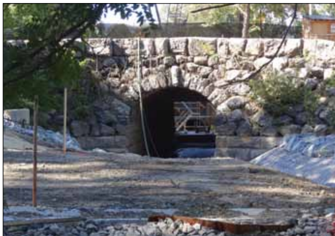
Fens Bridge on the downstream side at Ave. Louis Pasteur has been cleared of invasive plants. Flow of river has been diverted around the Upper Fens Pond.
