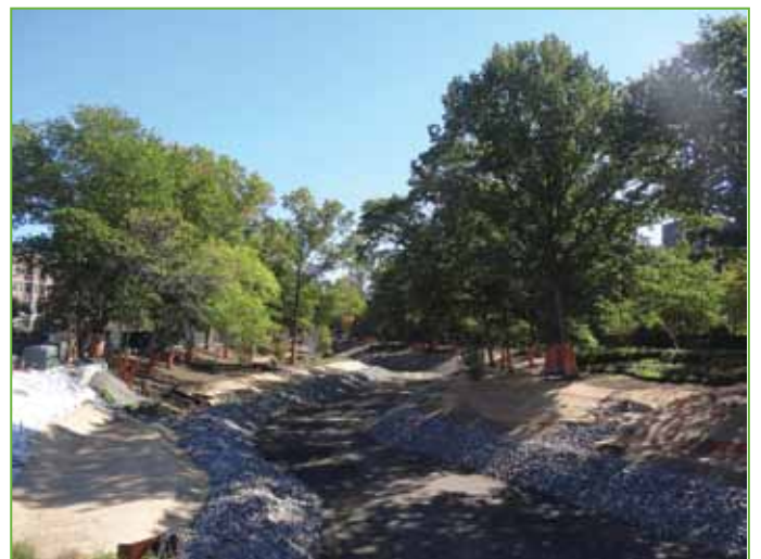
View of Upper Fens Pond from jughandle road at Brookline Ave., soon to be eliminated. Sediment has been removed, channel defined, and shrub and tree planting is in process. Over 8,000 shrubs and 200 trees will be planted in the Phase 1 area.
