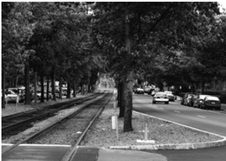
Newly set curb extension temporarily filled with existing large gravel, near Englewood Avenue. Photo by Judy Wong
