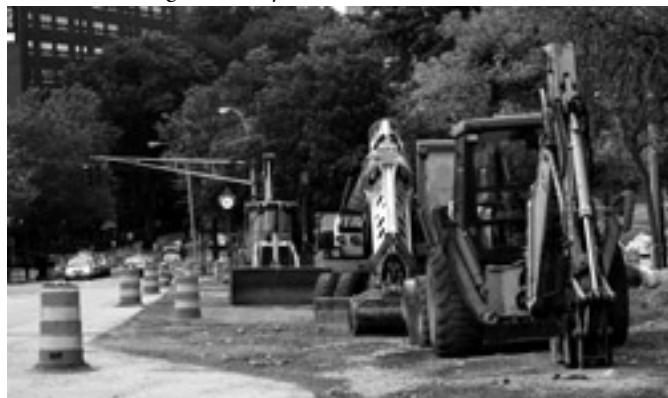
Large construction vehicles ripping out pavement near Englewood Avenue. Photo by Judy Wong
