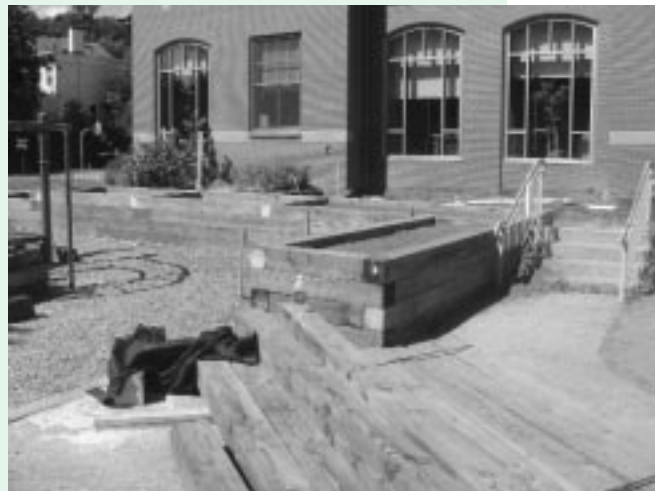
New outdoor seating and planting beds, under construction at the New Lincoln School.
