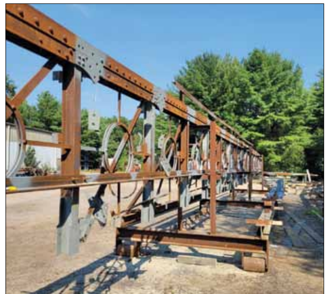
Below and at left: Welding, re-enforcing, sandblasting, priming and painting of the main span.
